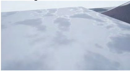
Figure 6 Puddle formation on plain surface
