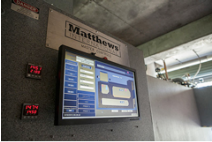
Figure 5: Control panel of the cremator
